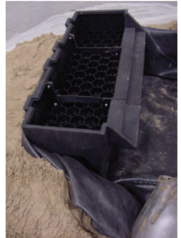
The liner goes under the spillway and wraps up the back and ends.
