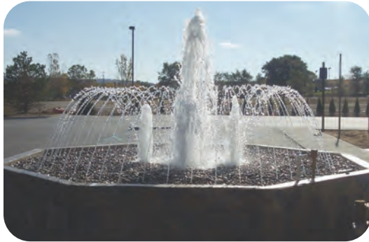
Nozzles can be installed vertically or at an angle. This feature has smooth jet nozzles surrounding frothy nozzles.
