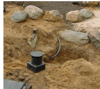
Use leftover dirt from reservoir to build up berm around top of waterfall if needed
